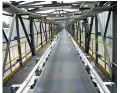
CESC HALDIA - Coal Handling Plant 2x300 MW TPP
